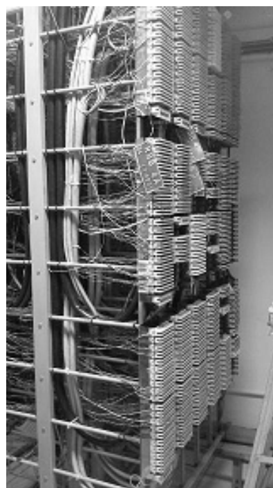
Gambar 12. Main Distribution Frame
